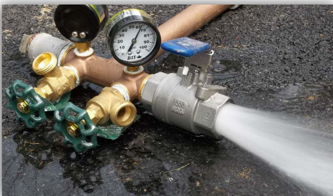
Redundant Potable Water Supply
