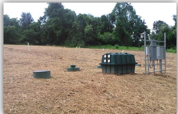
Wastewater Treatment System & Drain-field
