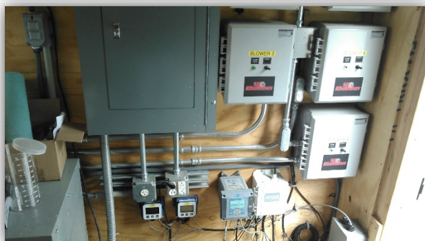
Controls & Remote Monitoring System
